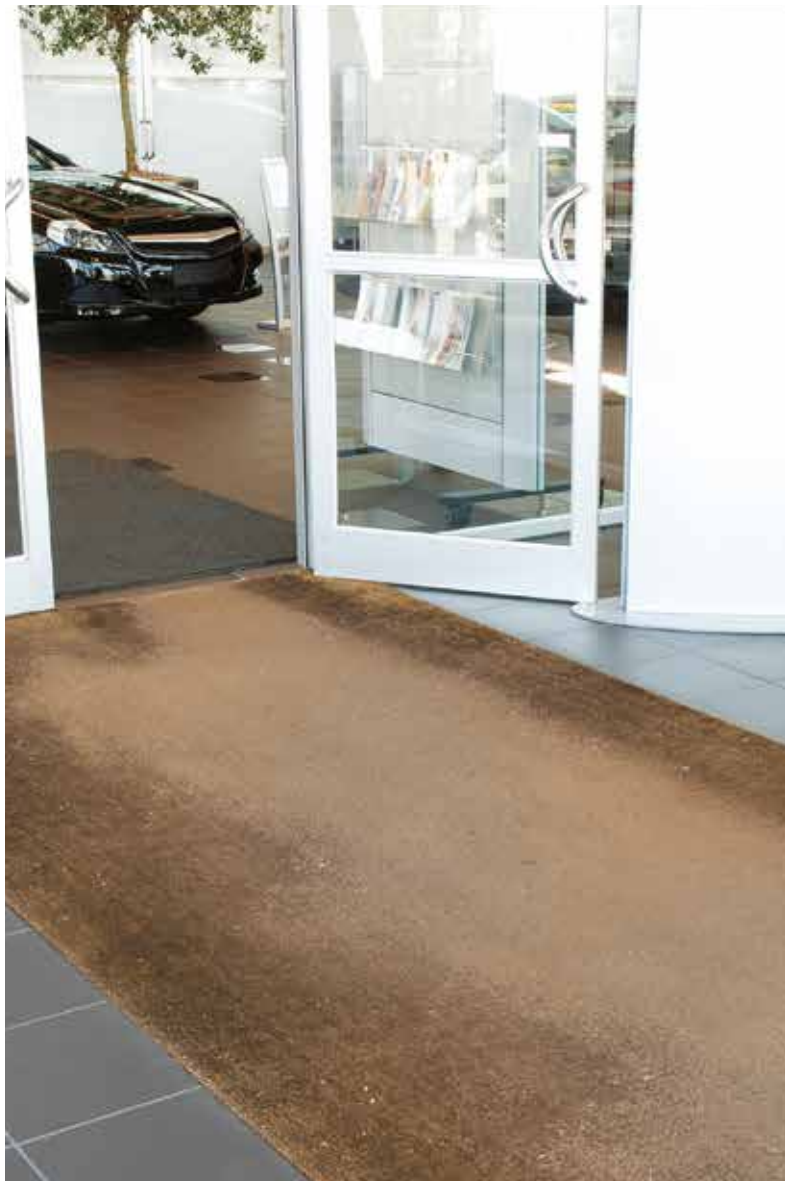
Entrance area with worn mat
